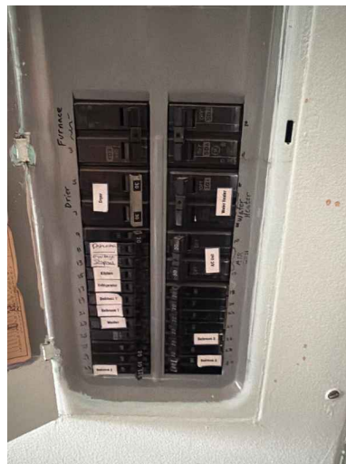
Interior Sub Panel
