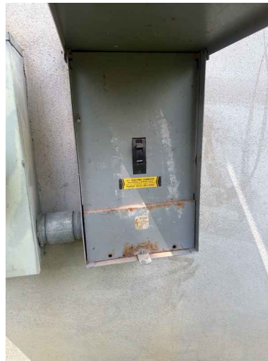
Main Electrical Panel
