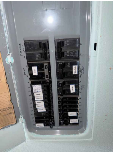
Interior Sub Panel
