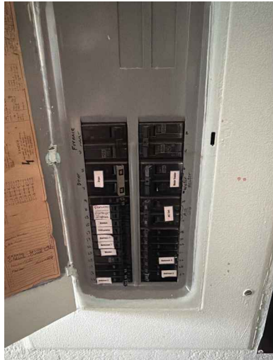
Interior Sub Panel
