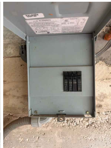
Exterior Sub Panel
