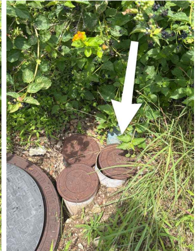
Pressure Reducing Valve
