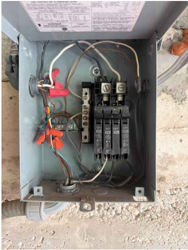
Exterior Sub Panel
