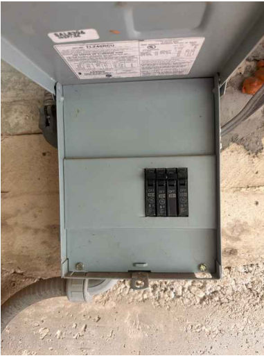
Exterior Sub Panel
