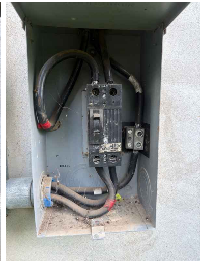
Main Electrical Panel
