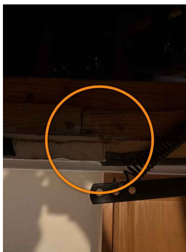
Frame appears to have been cut and altered
