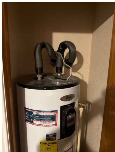
No service disconnect at water heater
