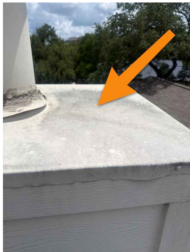
Stains from water pond
