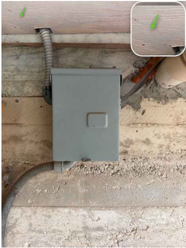
Exterior Sub Panel
