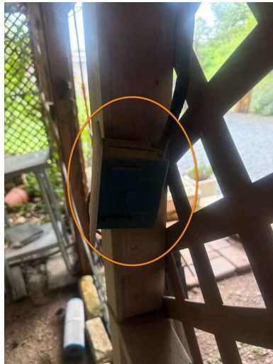
Non-weathertight junction box used at exterior, Back Of Home
