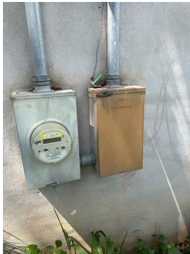
Main Electrical Panel
