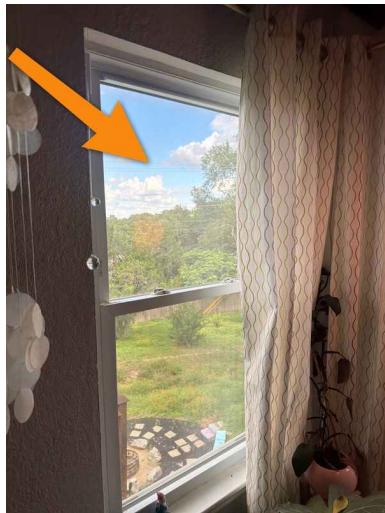
Upper sash balance damaged
