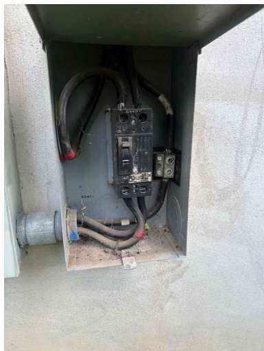
Main Electrical Panel
