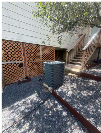
HVAC exterior condenser
